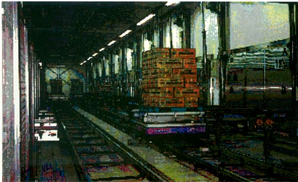
Servicing the new Netto DC at Koge, palletised goods are moved on a fully automated platform, designed by Daifuku.
